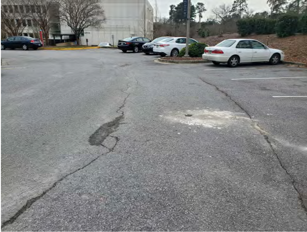
Photo 7: Longitudinal cracking near HA-2
