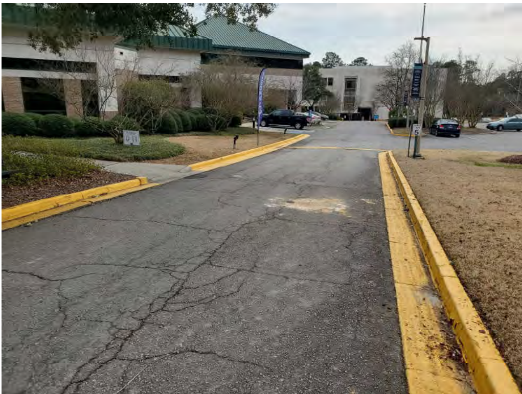
Photo 2: Moderate fatigue and longitudinal cracking near HA-1
