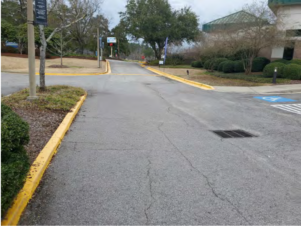
Photo 9: Slight longitudinal cracking near HA-3
