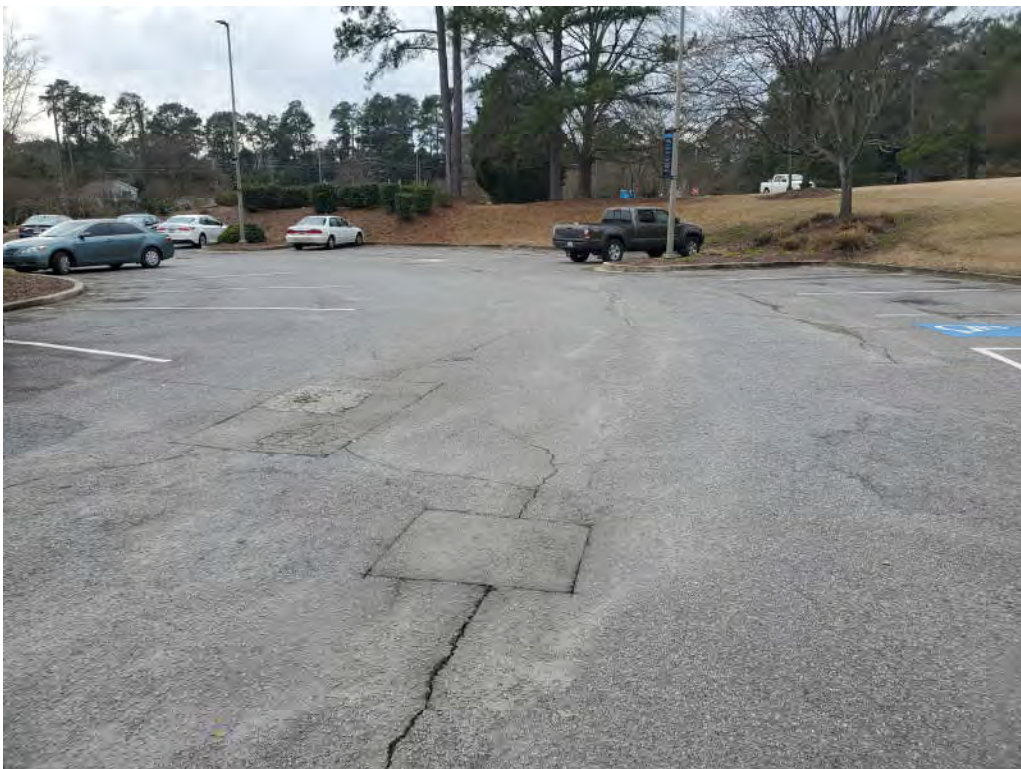
Photo 6: Longitudinal cracking HA-1 facing HA-2
