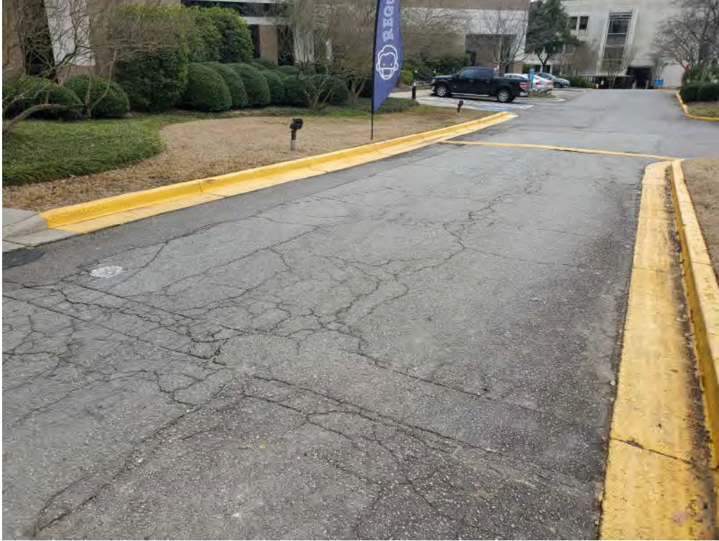
Photo 3: Moderate fatigue and longitudinal cracking near HA-1
