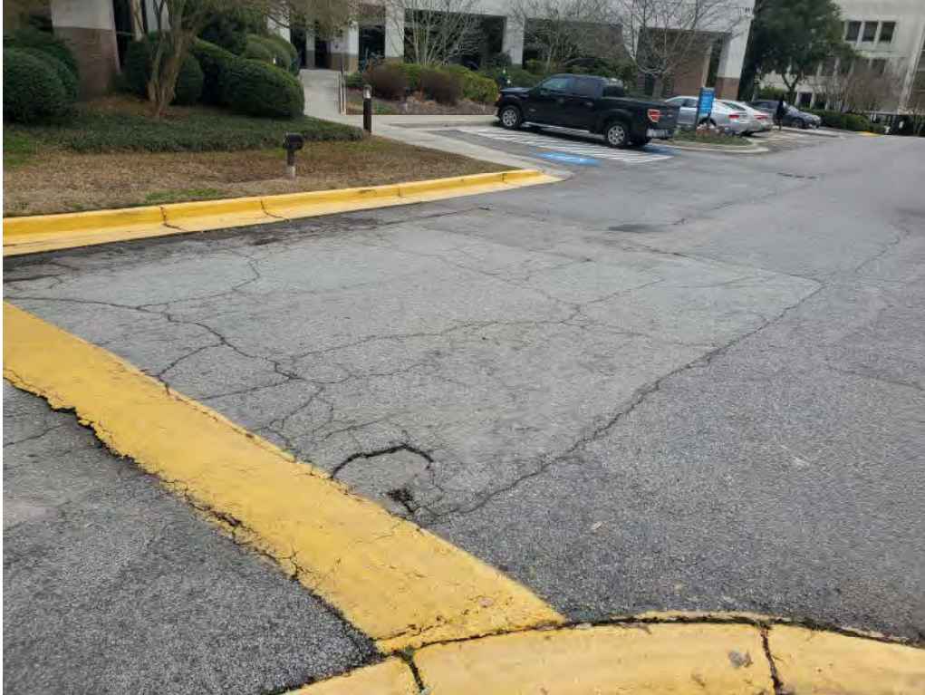
Photo 5: Slight fatigue cracking and moderate potholing
