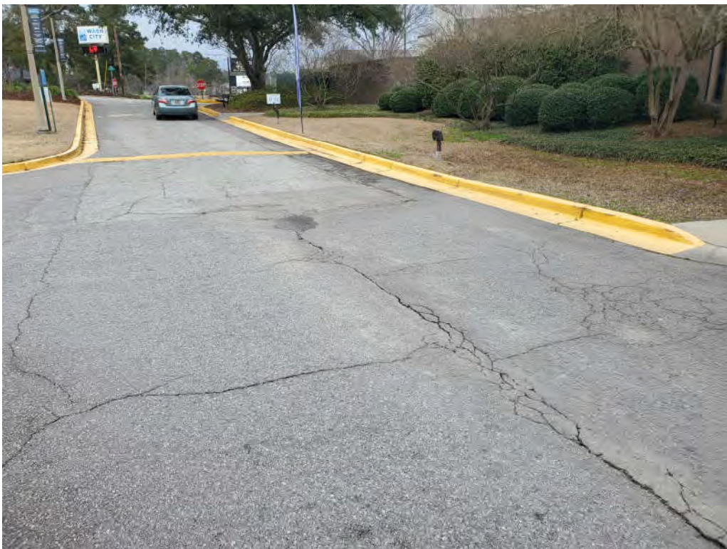
Photo 10: Longitudinal cracking and slight fatigue cracking near HA-3
