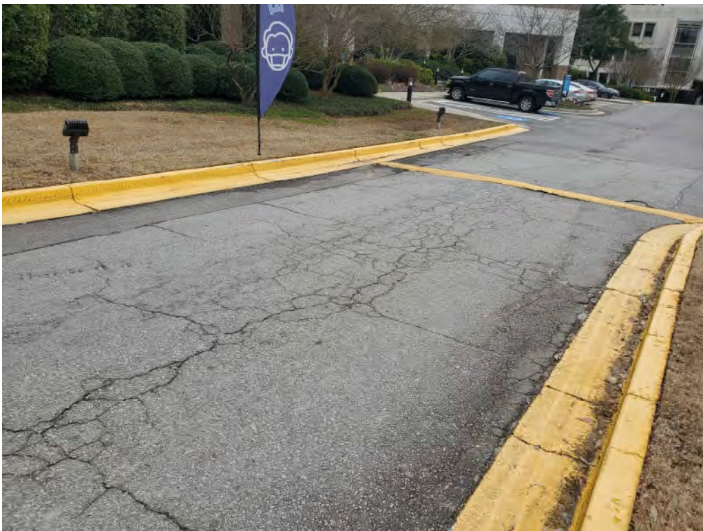
Photo 4: Moderate fatigue and longitudinal cracking near HA-1
