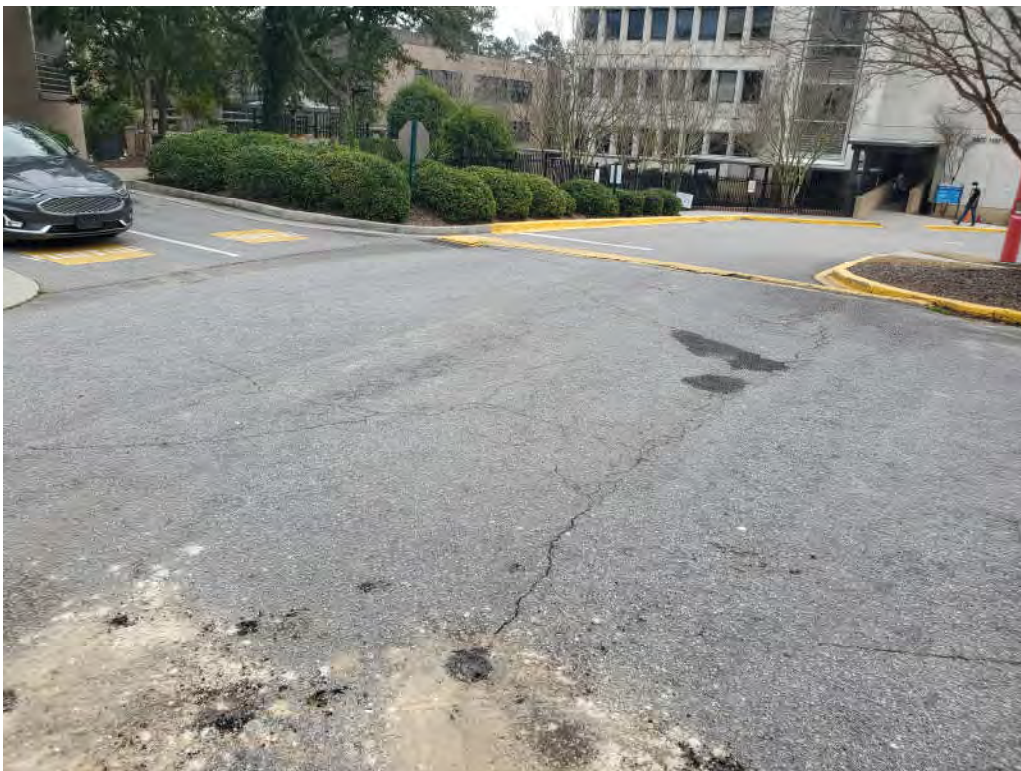
Photo 8: Longitudinal cracking near HA-3
