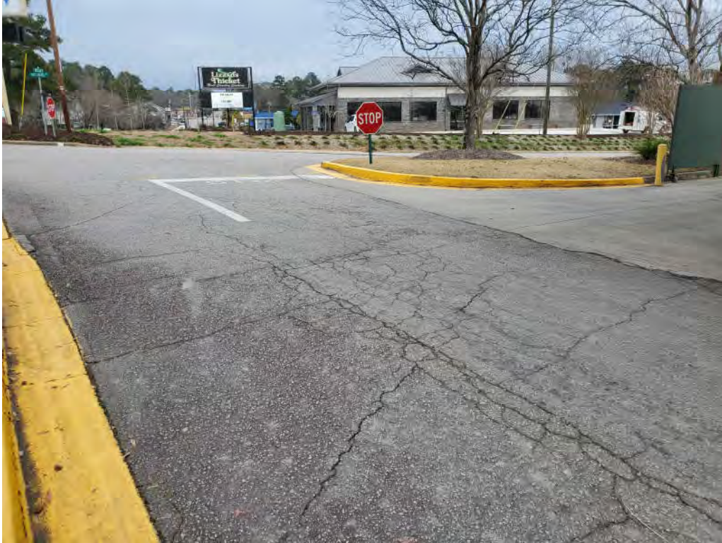
Photo 1: Moderate to severe fatigue cracking near HA-1
